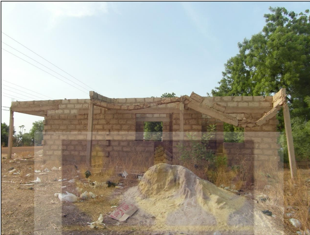
Plate 5.1 An uncompleted structure built with substandard materials in Mangu
