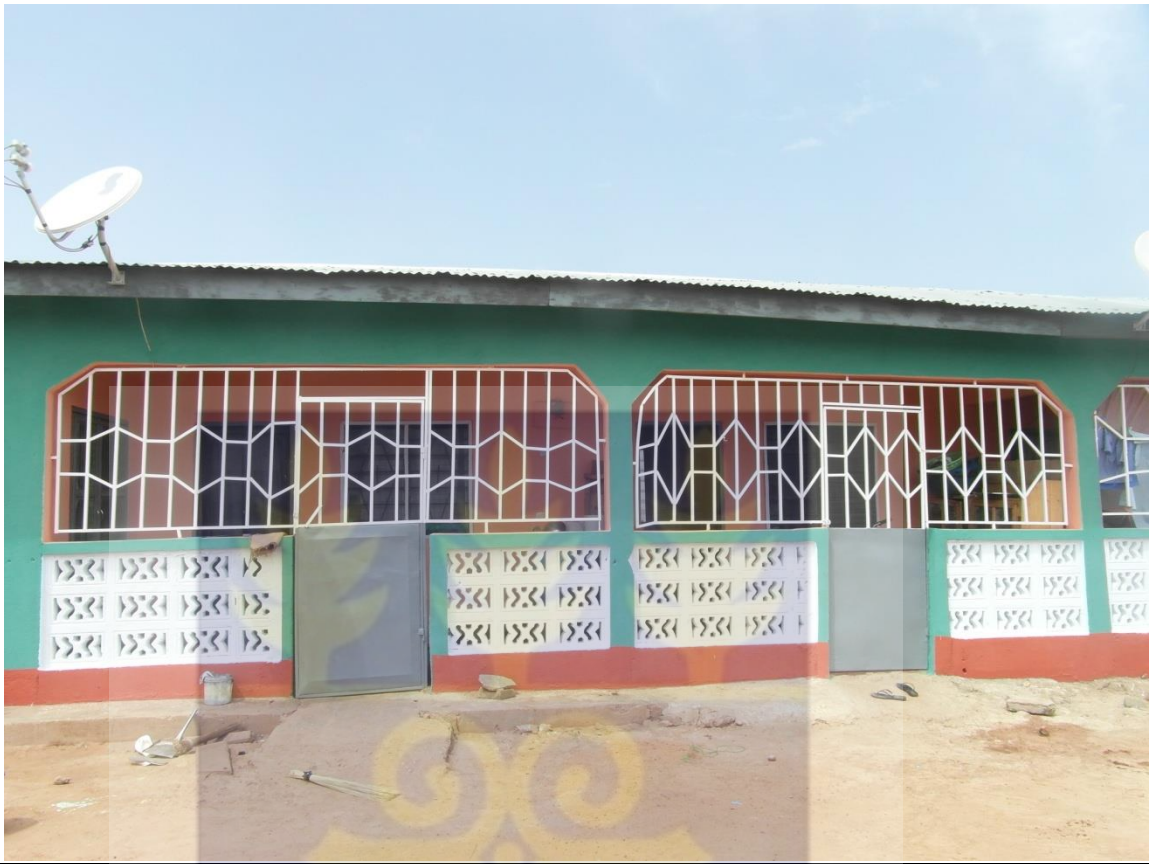
Plate 6.1 A respondent's house protected with burglar proof to prevent thieves from entering
