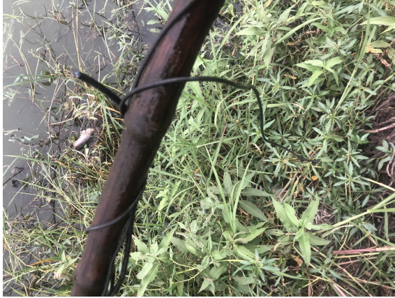
Figure 6. 33 Sensor Cables Damage
