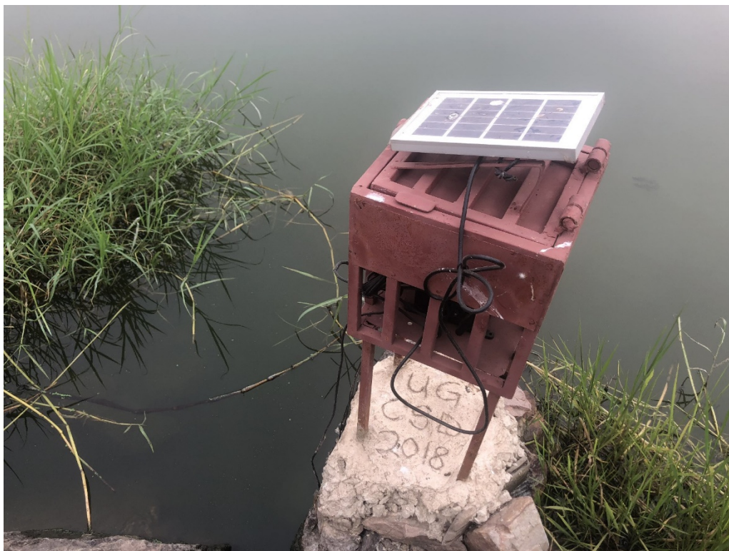
Figure 6. 28 Externally mounted solar panel for energy harvesting in freshwater
