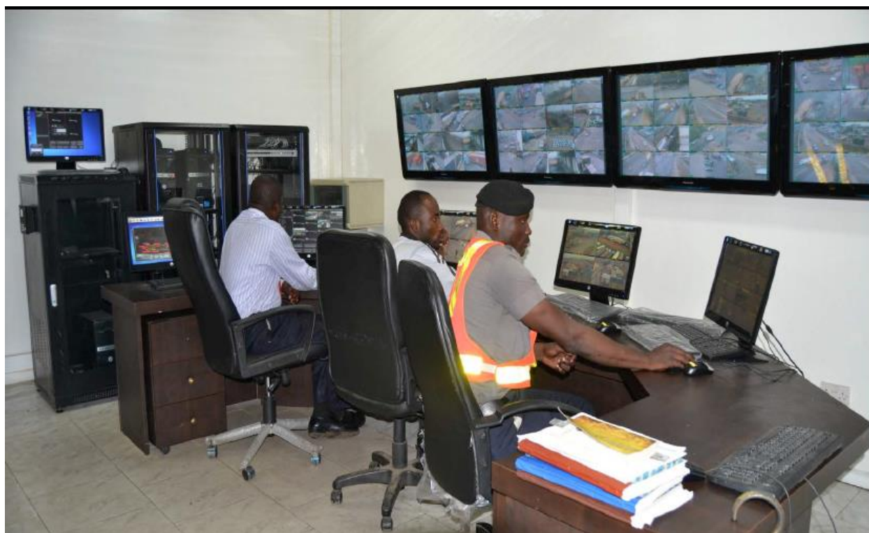
Figure 18: GPHA CCTV Control Room
