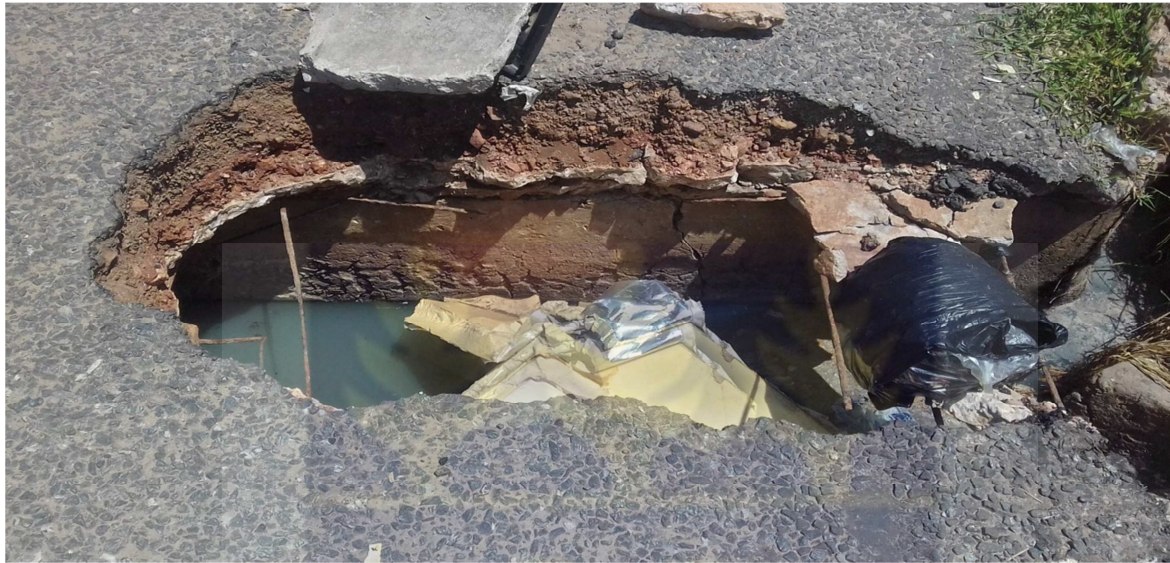
Plate 4.7: A bridge at Fisheries destroyed by Floods
