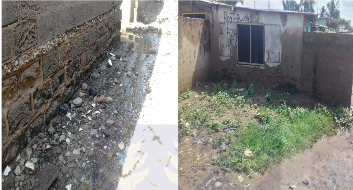
Plate 4.4 Walls of buildings destroyed by floods in Adzeman and Kenan Factory
