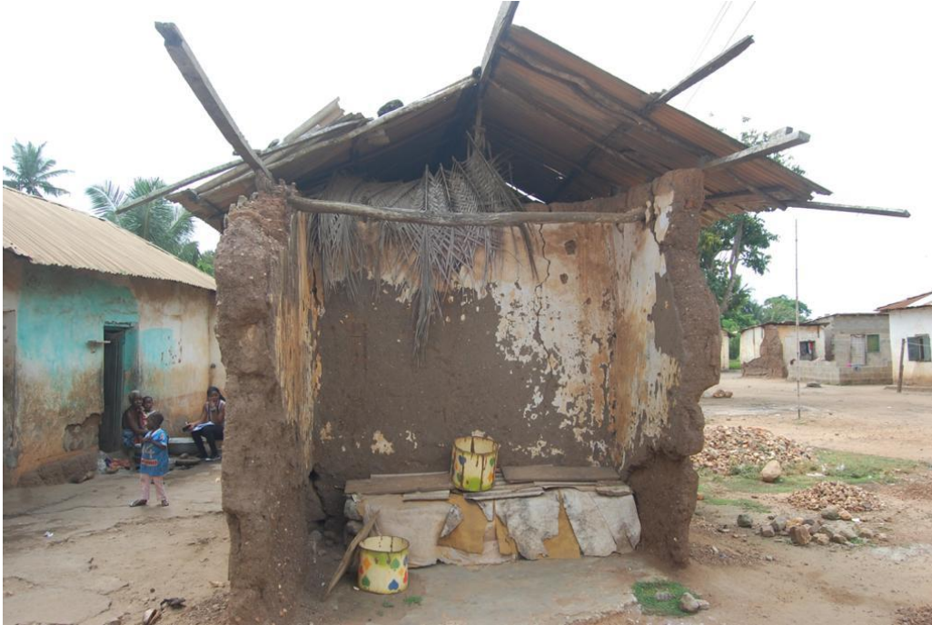
Figure 4.2-11: Mud house in ruin. Source: Author
