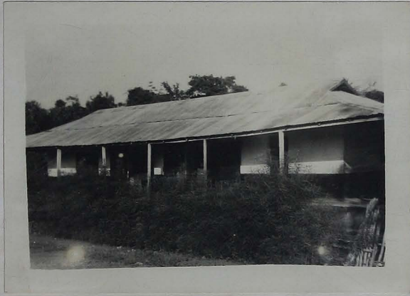
Old roadside stores and cocoa sheds converted into classrooms for the Presbyterian Primary School.
