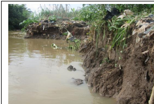
Plate.5.3A: Evidence of cantilever bank failure along the bank of the Oda River at Asaago – Kumasi.
