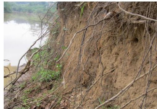
Plate.5.3B: Evidence of cantilever bank failure along the bank of the Birim River at Akim – Oda.
