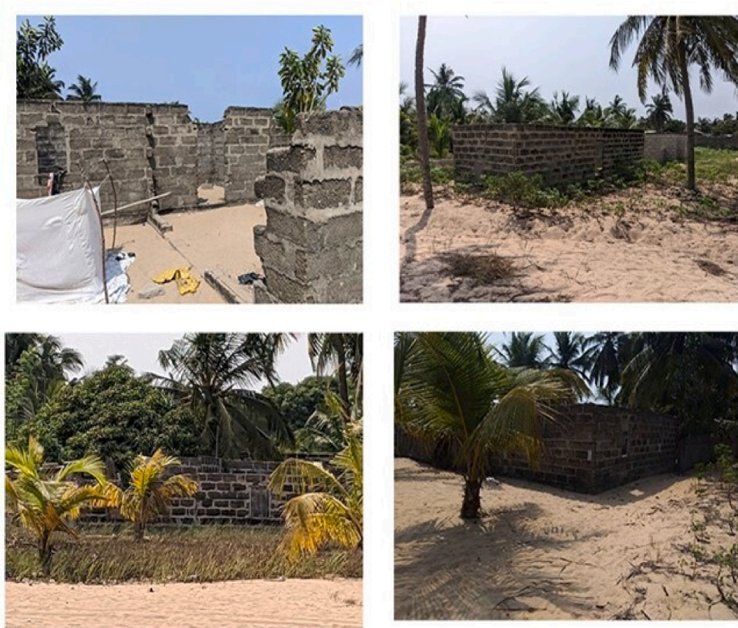
Fig. 5. Damaged building caused by 2021 keta coastal flood. Source: Author 2023
