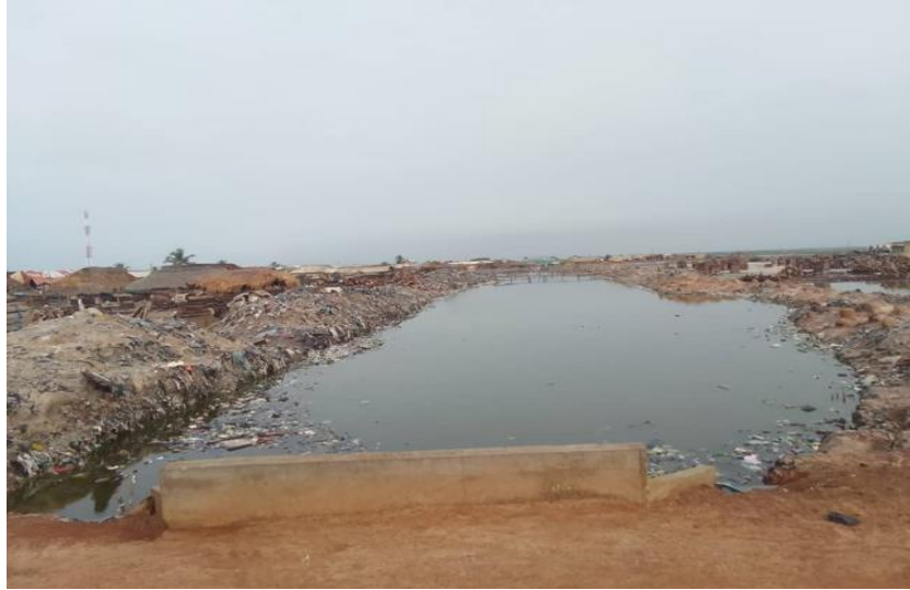
Community drain in Akplabanya that was built to relief coastal flooding and rainfall.
