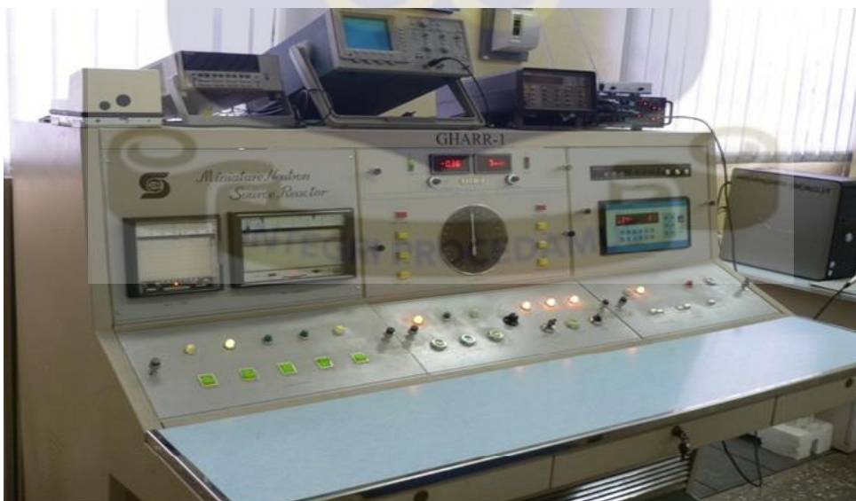
Figure.2.10 b Control Console
