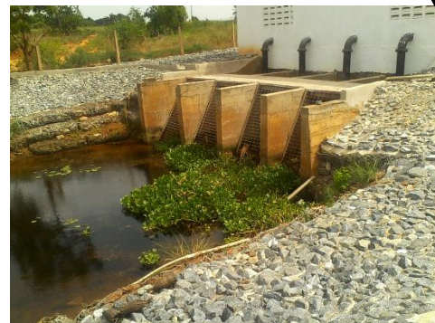
Plate 4. 7: Pump station at Dordoekorfe
