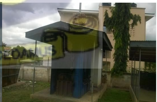
A broken-down Incinerator
