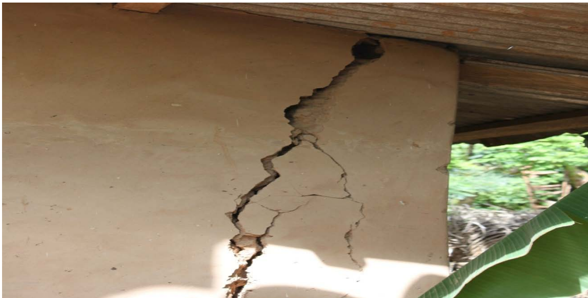
Plate 32: Cracks in a 4-year old building at Odugblase about 300m from GHACEM quarry
