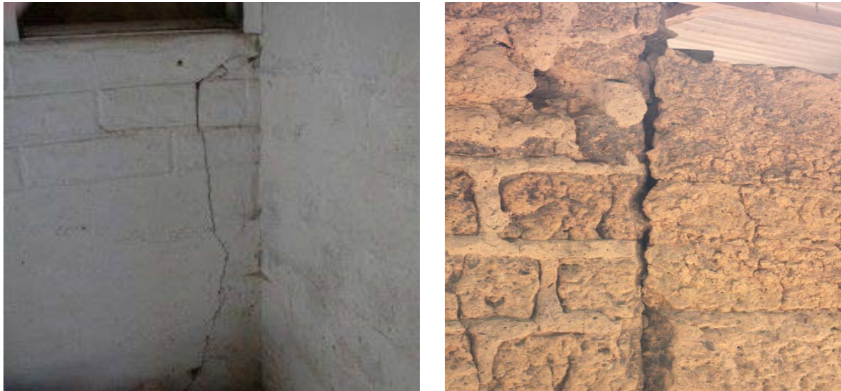
Plate 15: Blasting causes cracks in buildings
