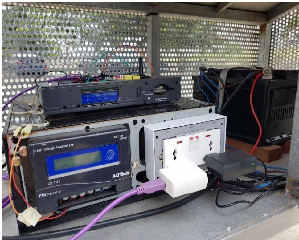
Illustration 18: Inside the multifunction workstation
