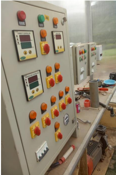
Plate 24: Electric control panel
