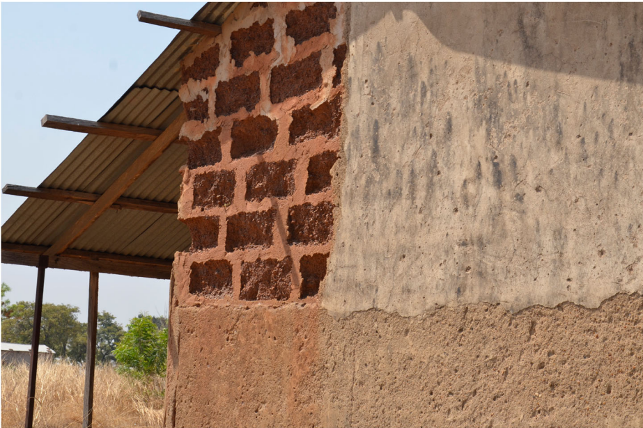
Figure 6. Eroding wall surface. Photograph taken by the author, 2019.
