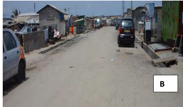
After street and drain construction, Glefe Image B taken during transect walk, 2017
