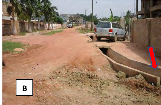
Uncompleted drain, Ogbojo
