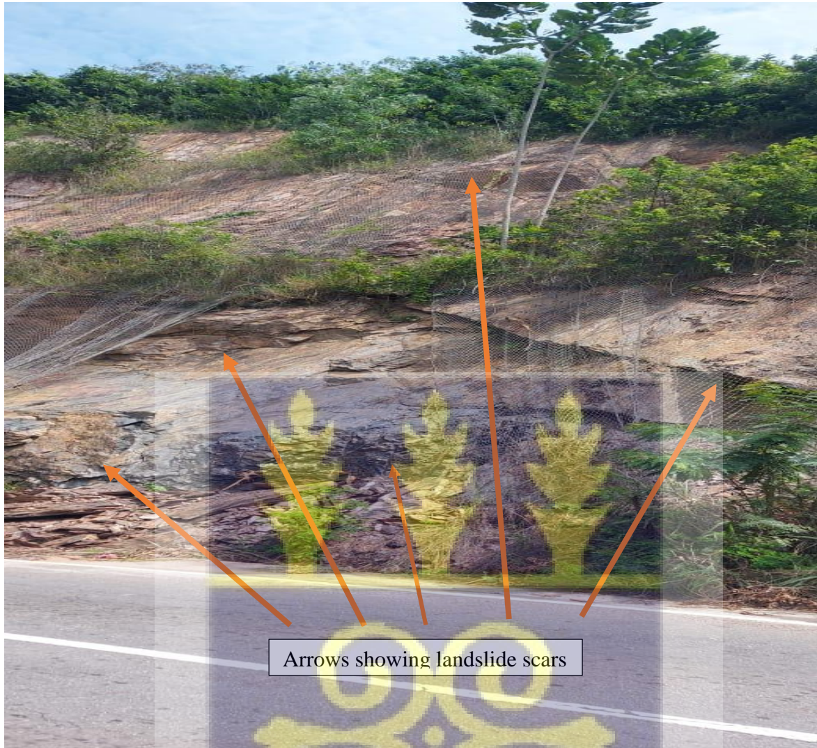
Plate 3: Scars from landslides along the Peduase road
