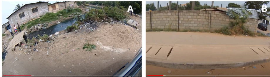
Fig. 8. Comparing similar sized gutters in two different communities. 'A' show an open drain in a lower income community and 'B' shows a drain in a middle-income community.
