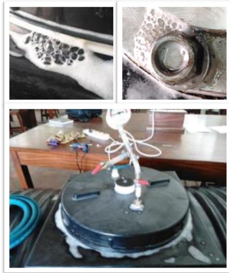
Figure 4-3: Gas leakage tests showing escaping gas through soap bubbles
