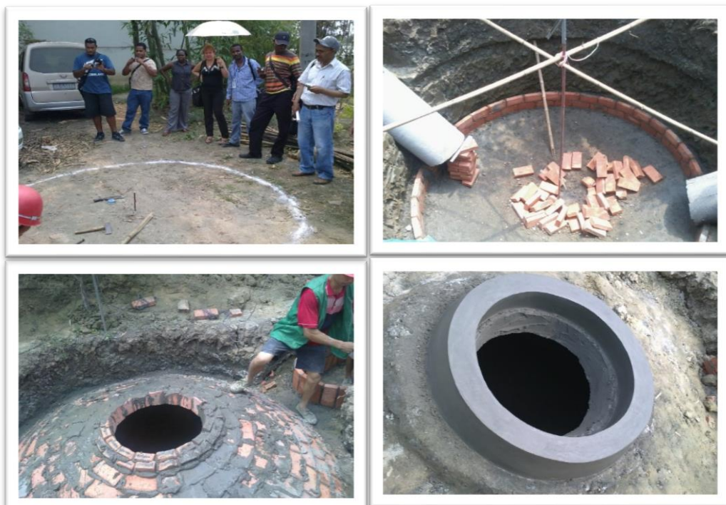
Figure 2-8: Stages of construction of a Chinese brick fixed dome digester Source: (BIOMA P. R. C., 2013)
