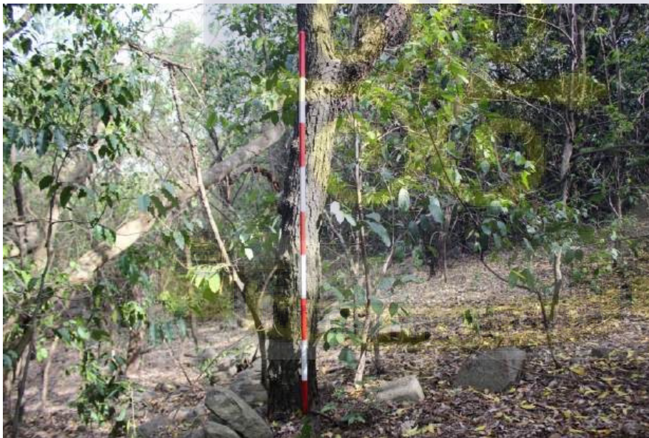
Figure 31: A completely damaged retaining wall (photo by Odarkor Ankrah-Addison, 12/04/2023).
