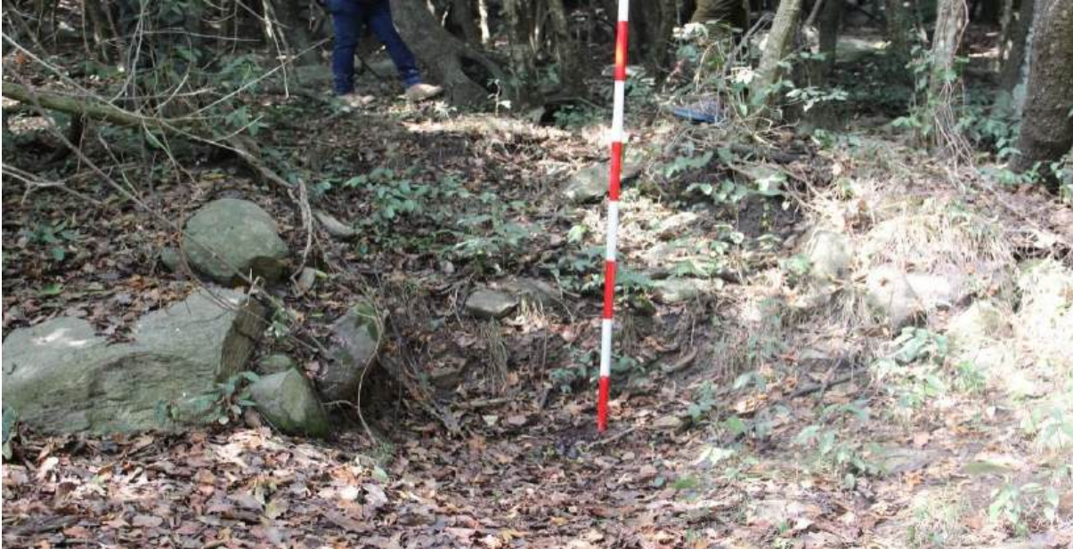
Figure 17: A Damaged retaining wall at Manya Hill (photo by Odarkor Ankrah-Addison, 14/04/2023).
