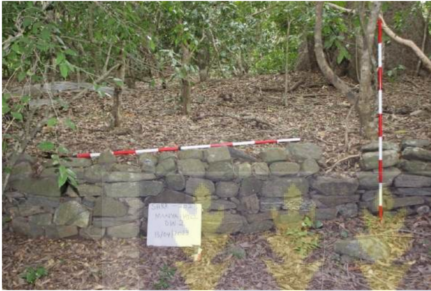
Figure 22: A partially destroyed defense wall (photo by Odarkor Ankrah-Addison, 13/04/2023).
