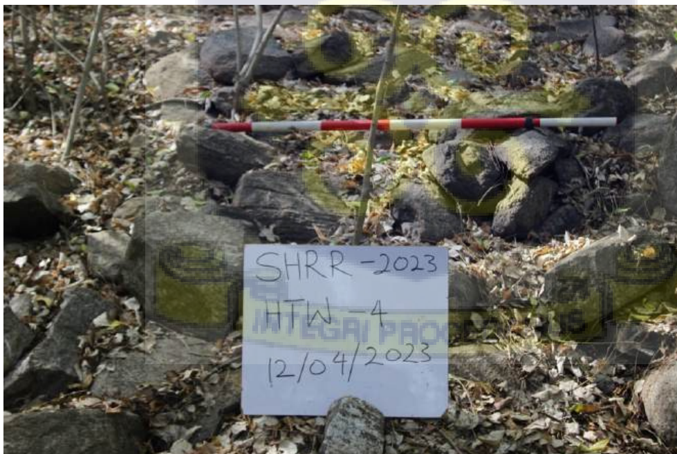
Figure 29: A damaged building foundation at Hioweiyi site (photo by Odarkor Ankrah-Addison, 12/04/2023).
