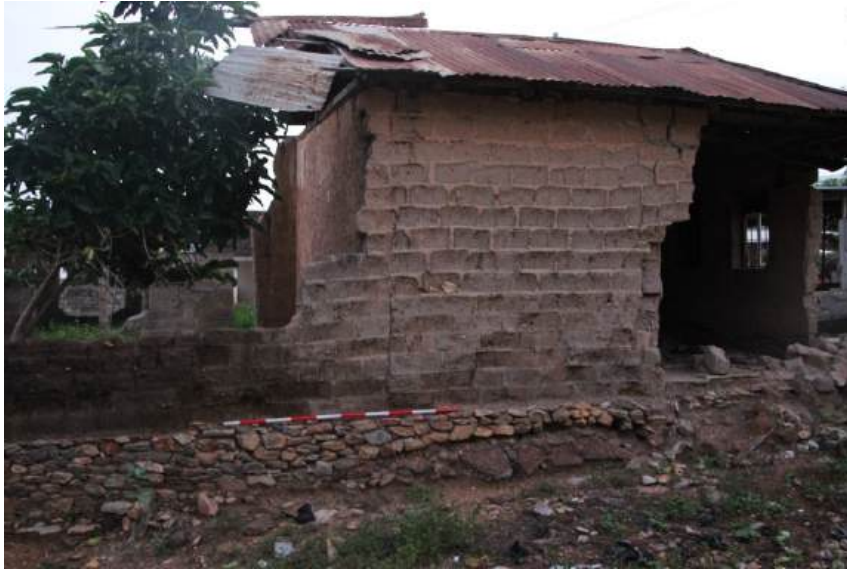
Figure 7: An old, abandoned building at Agomeda (Picture by Odarkor Ankrah-Addison 28/06/2023).
