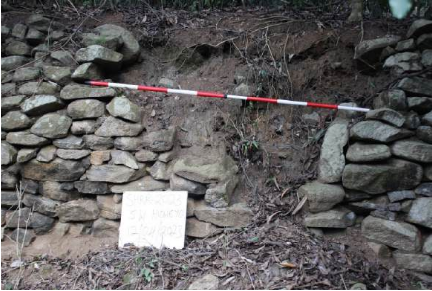
Figure 34: A partially damaged defense wall (photo by Odarkor Ankrah-Addison, 12/04/2023).
