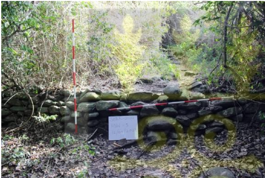
Figure 33: A partially destroyed defense wall (photo by Odarkor Ankrah-Addison, 12/04/2023).
