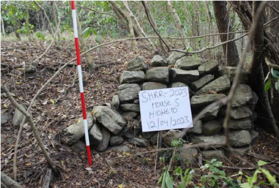
Figure 37: A partially damaged building foundation (photo by Odarkor Ankrah-Addison, 12/04/2023).
