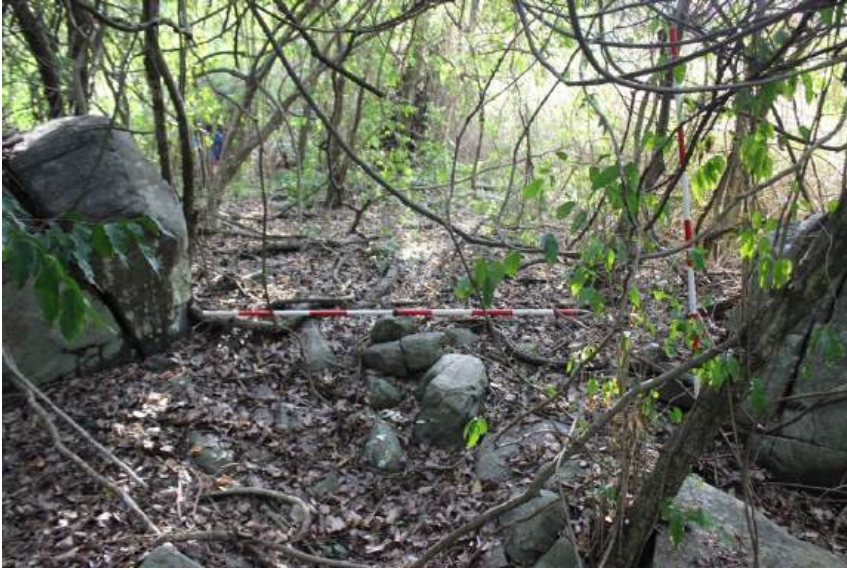
Figure 32: A completely damaged retaining wall (photo by Odarkor Ankrah-Addison, 12/04/2023).
