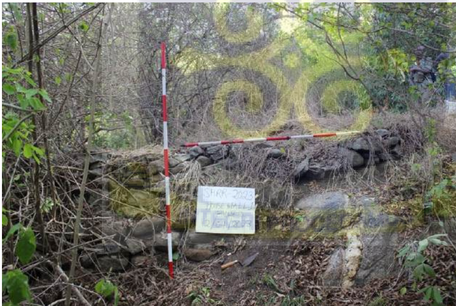
Figure 36: A partially damaged building foundation (photo by Odarkor Ankrah-Addison, 12/04/2023).
