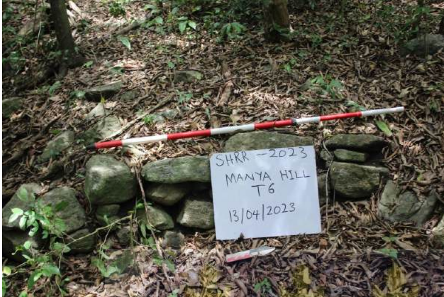
Figure 23: A partially destroyed retaining wall. The rubbles that make up the wall are scattered around. (photo by Odarkor Ankrah-Addison, 13/04/2023).
