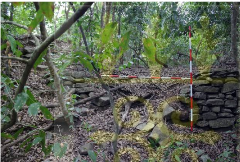
Figure 38: A partially damaged building foundation (photo by Odarkor Ankrah-Addison, 12/04/2023).
