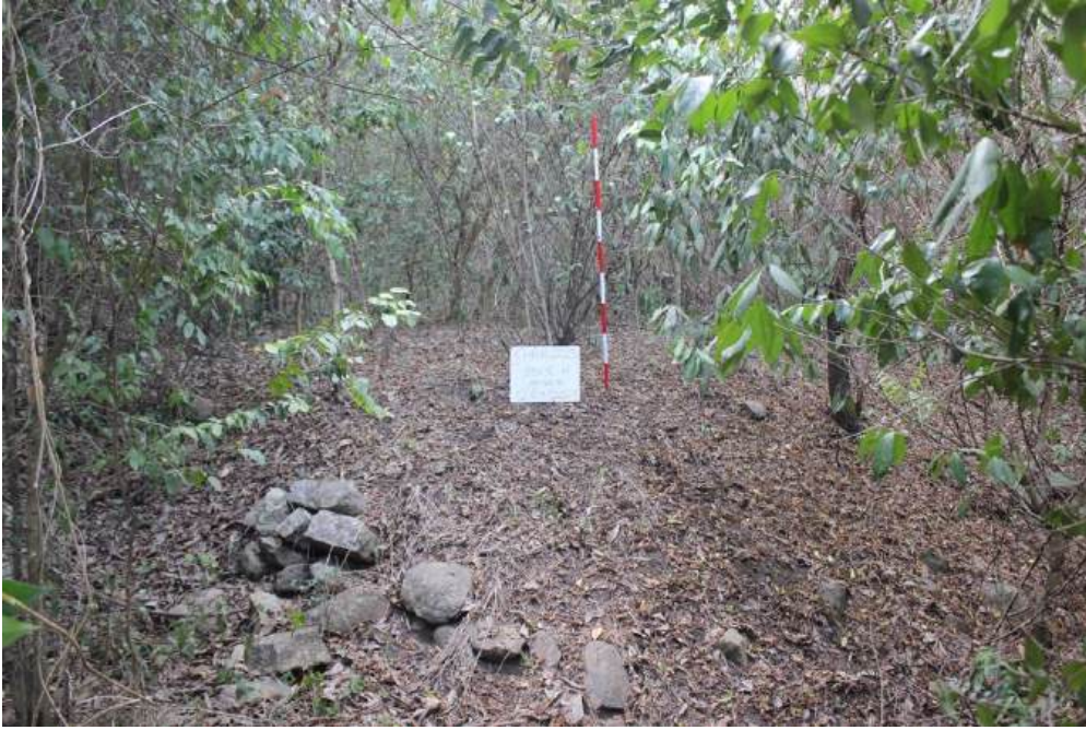
Figure 30: A completely damaged building foundation (photo by Odarkor Ankrach-Addison, 12/04/2023).
