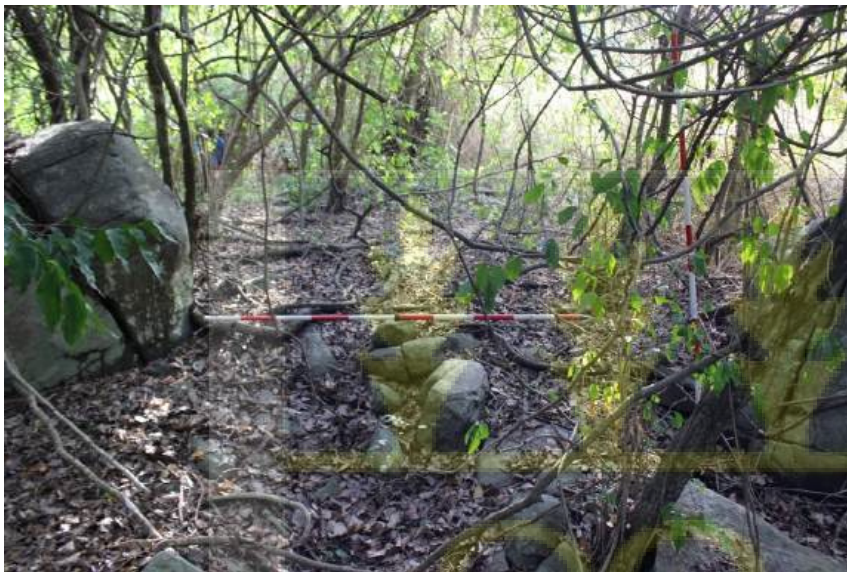
Figure 35: A damaged retaining wall (photo by Odarkor Ankrah-Addison, 12/04/2023).
