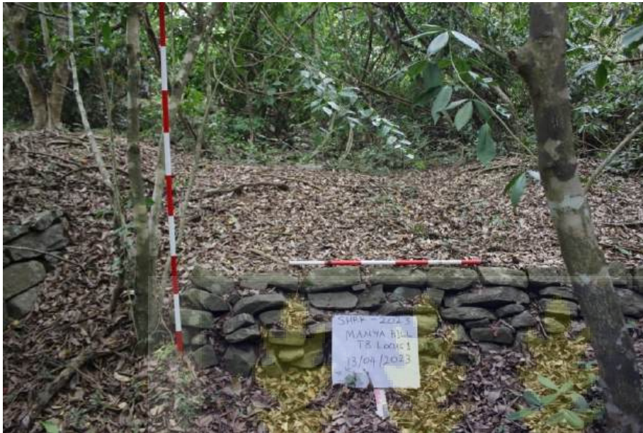
Figure 24: A partially destroyed retaining wall. The tree growth within the wall has caused most of the pellets to move from their original position. (photo by Odarkor Ankrach-Addison, 13/04/2023)
