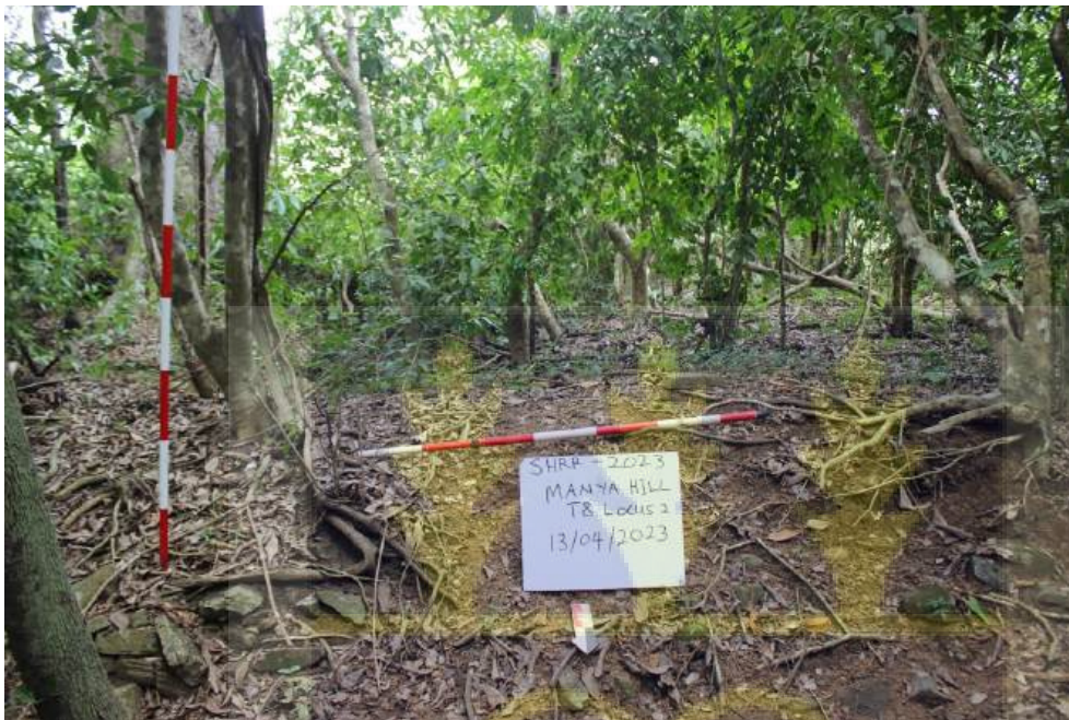
Figure 25: A destroyed building foundation (photo by Odarkor Ankrah-Addison, 13/04/2023).
