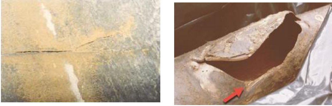
Figure 1.1: Thermal fatigue failure [8]
