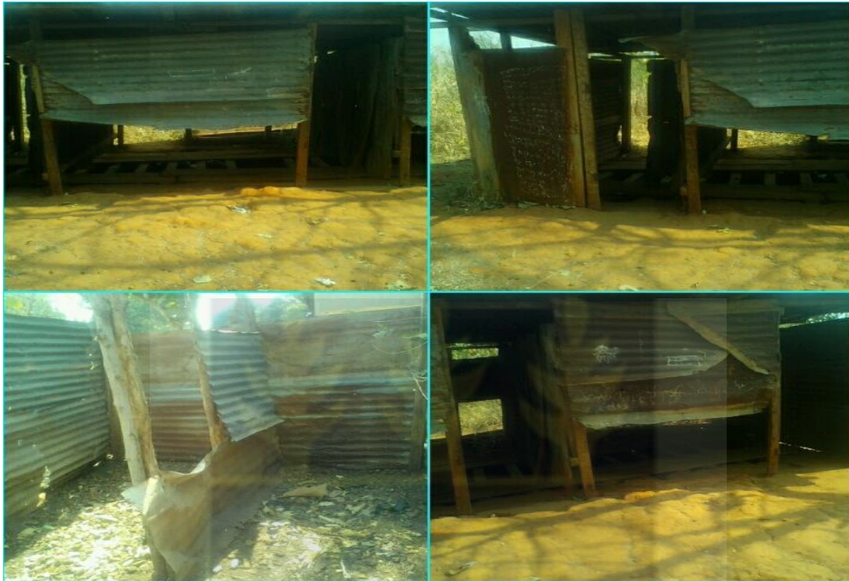
Plate 4. 3: Conditions of Toilets and Urinals (bottom left) at Ankamadoa RC Primary
