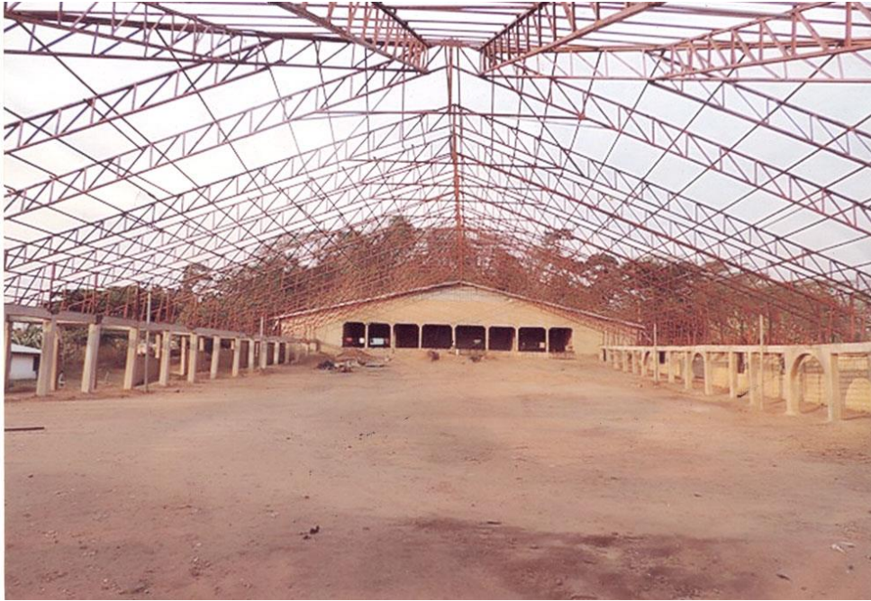
Picture 4: A church auditorium at Abasua centre 250x120ft under construction construction (August 17, 2014)
