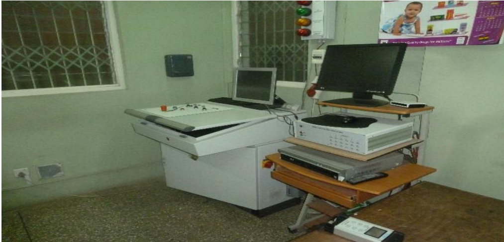
FIG. 3.12: Radiation Monitoring Room
