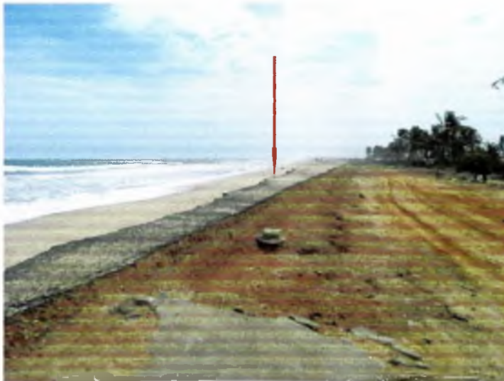
Figure 5. 6 Destruction by Erosion at (a) Blekusu and (b) Atorkor
