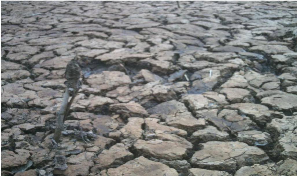
Plate 4: Cracked unremediated land surface at Kalaba community due to oil spill impact.
