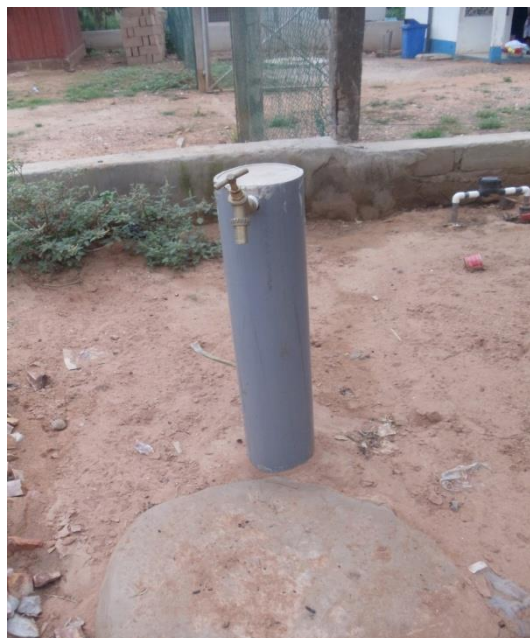
Picture 4: Community Stand Pipe
