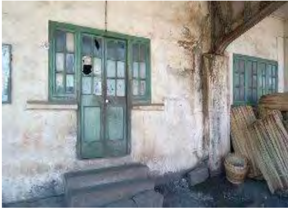
Field Survey 2018. Dilapidated Nsawam railway station
